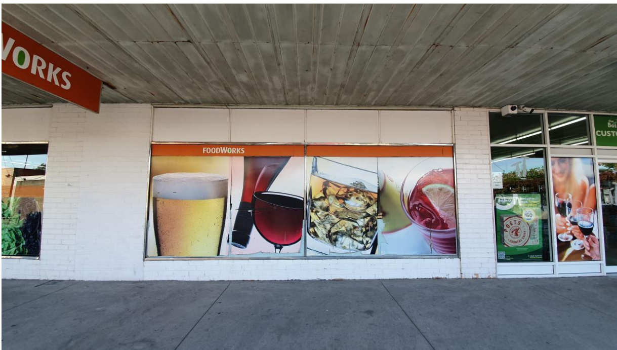
Image 16: the façade has undergone subsequent alterations since the 1964 works. More recent changes include the installation of new glazed window / automatic doors.
